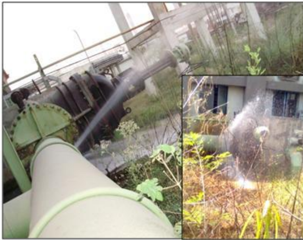
Leakage at pipe to aerator
