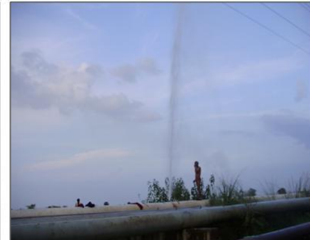
Leakage jet at pipe
