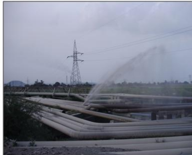
Burst pipe leakage jet
